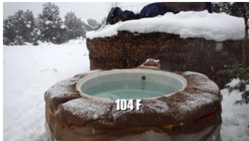
Compost-Powered Water Heater provides Free heat for the Hot Tub and helps me grow organic food. (137)
